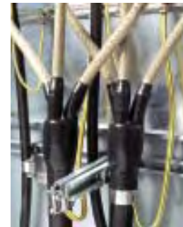
Mounting two 3-core cables with screen connection kits and three 1-core cables
