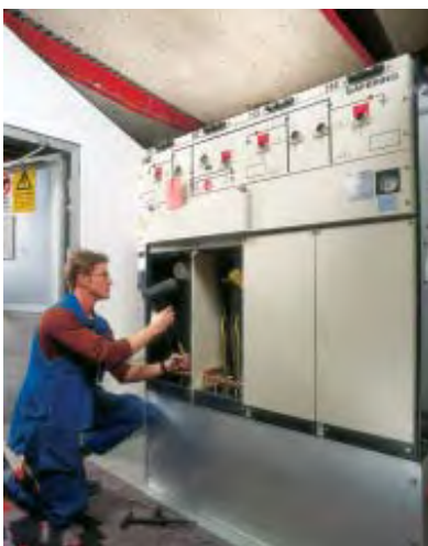
SOC 630 A in ABB SafeRing, Sweden.
