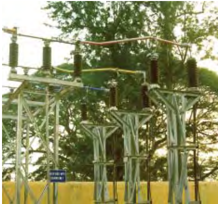
APED 72 kV, India.
