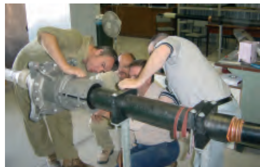
APECB assembled horizontally on the ground before lifted it into place, Australia.
