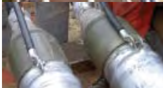
SMPGB 170 kV with sheath sectionalizing, Ireland.
