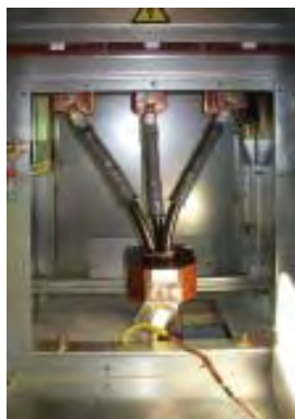
SOT 12 kV in a switchgear box, Sweden.
