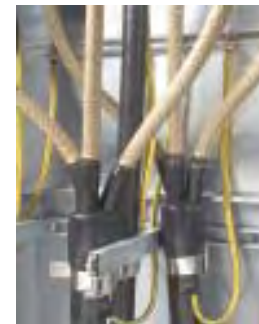
Mounting two 3-core cables with screen connection kits and three 1-core cables
