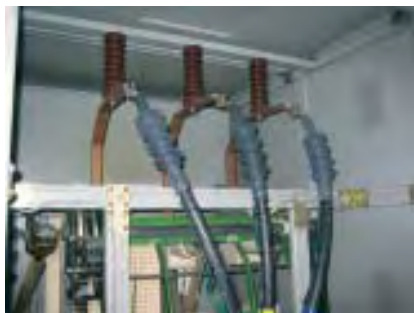
SOT 24 kV connect switchgear to transformer.
