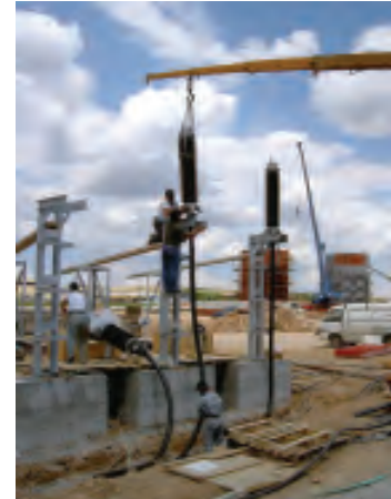
APECB with porcelain insulator, assembled horizontally on the ground before lifted it into place, Greece.
