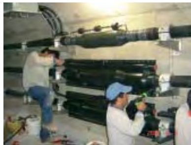
SMPGB 170 kV with sheath sectionalizing, Mexico.
