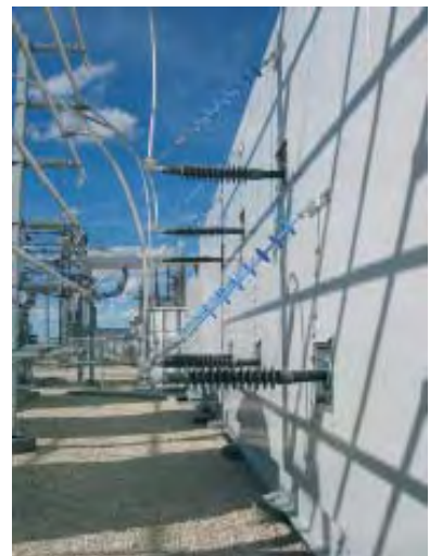
APSEA installed on the wallbushings, USA.
