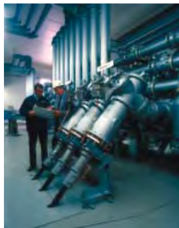
APEGA 110 kV at GIS, Finland.
