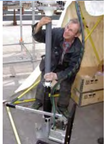
JS 72 kV installation, Sweden.
