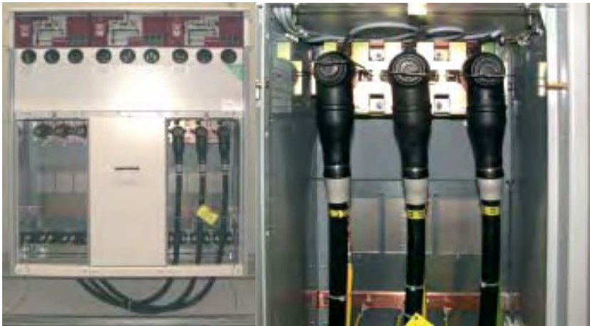
SOC in Eaton switchgear, Sweden.
