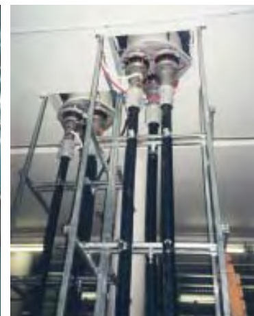
APEGA 170 kV at GIS, Australia.
